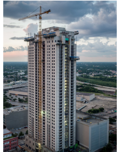
Market Square Tower rises above downtown Houston in this June 2016 aerial photo.
