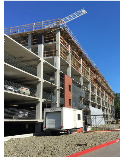
The parking deck is being built using post-tensioned cast-in-place concrete by Ferguson Construction in Bellevue, WA.
